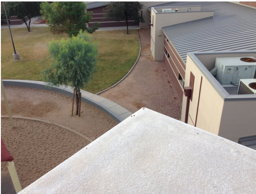
Holes along the gravel stop due to Wood Peckers.
