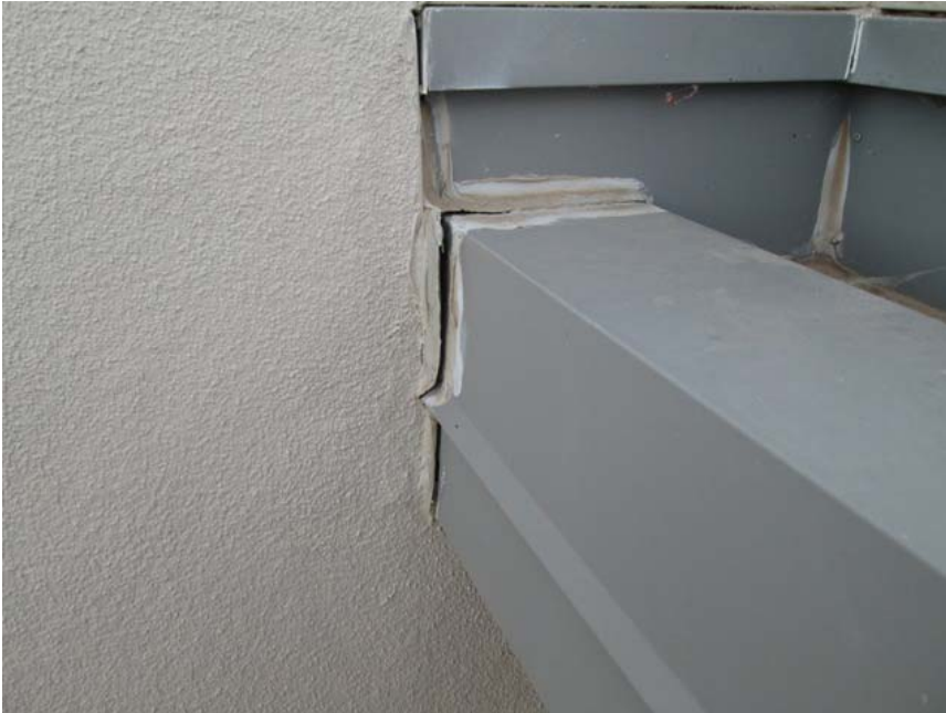
Perimeter voids at copings
