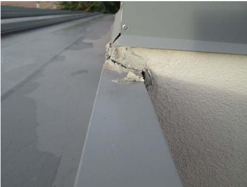
Perimeter sealant voids at metal roofing
