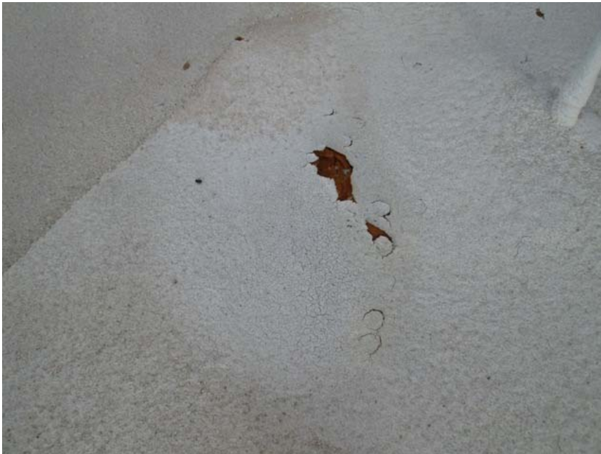
Blisters at south roof
