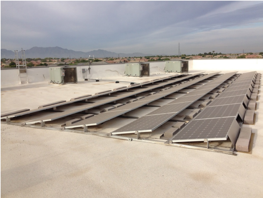
PV arrays at MPR Roof
