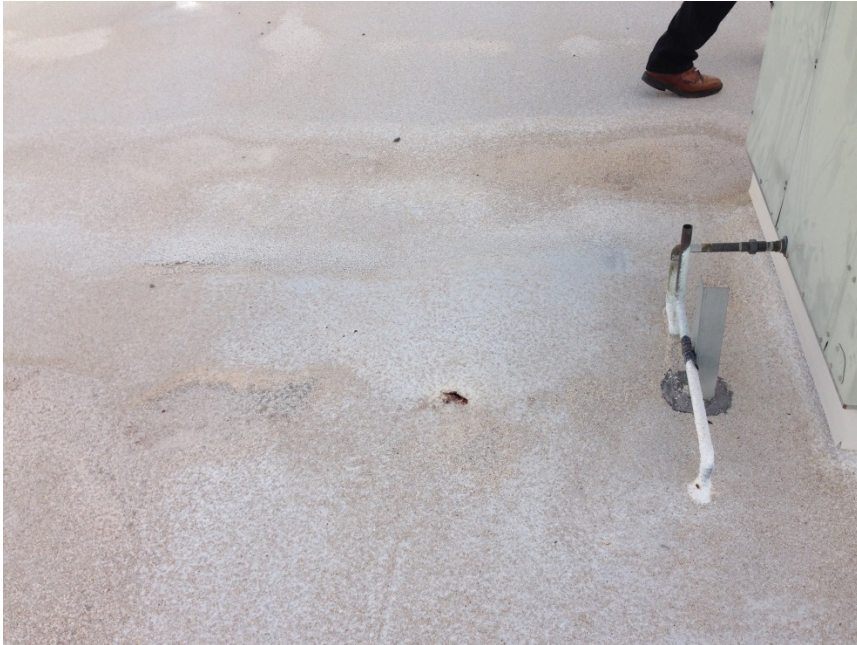
Large blister with tears in the coating at Admin Roof
