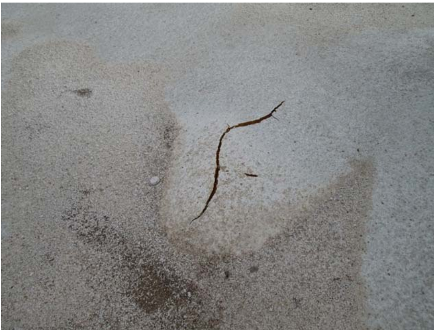
Fractured blister at SW Gym roof (1 of 10)
