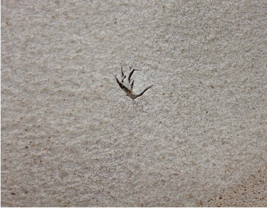
Fractures in cementitious coating
