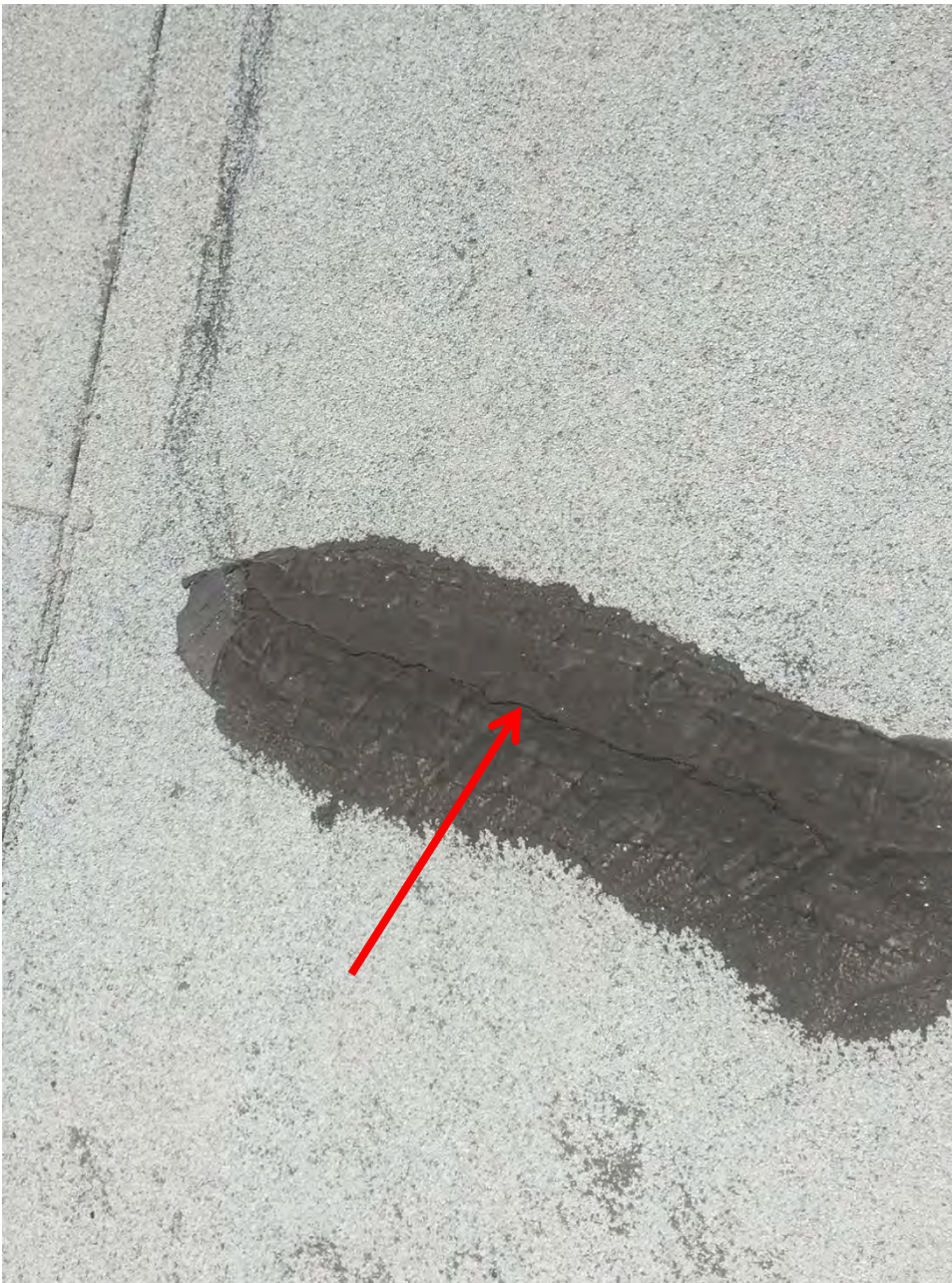
Overview photograph of buckling at the cap sheet that was patched incorrectly with roofing plastic. The plastic has shrunk and the crack has reopened.
