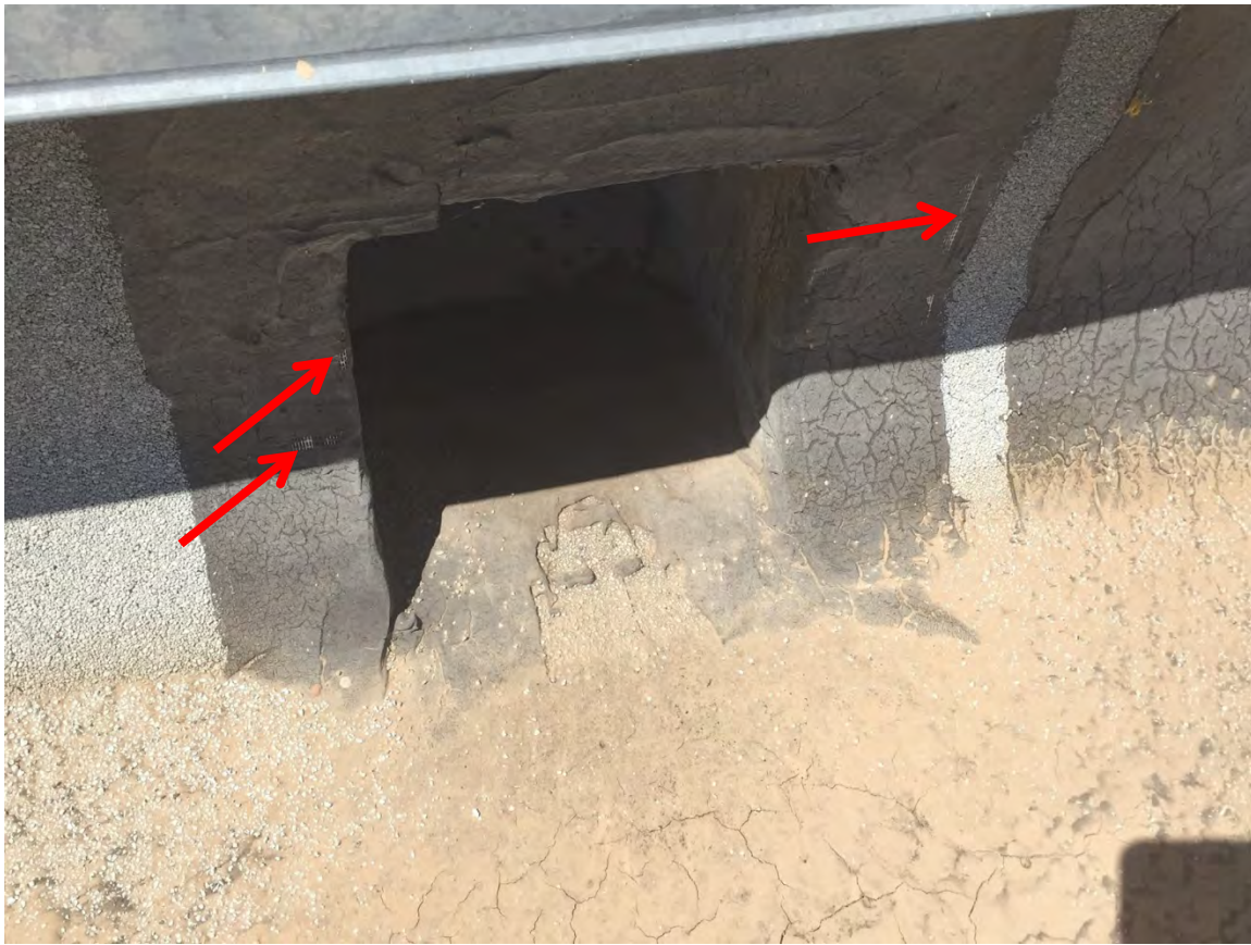
Roof scupper three (3) course repair has alligatored, cracked and shrunk allowing the fiber tape to become exposed (red arrows). This repair is no longer performing as intended. This condition was noted at isolated locations and not typical throughout.
